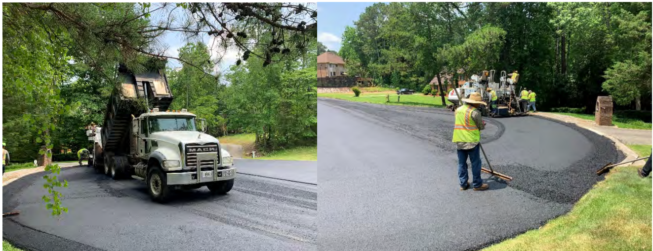
Resurfacing pictures: The City of Stonecrest's paving contract which SEI's Senior Inspector Mike Lehner oversaw.
